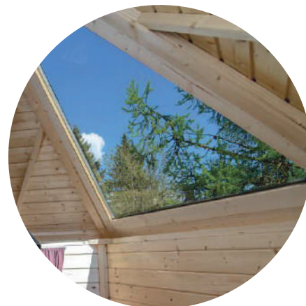
Roof window is not opening. The glass is clean and tempered, 8 mm thick
